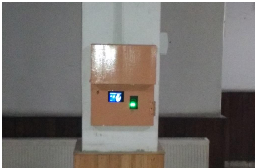
One of the two Biometric Attendance Machines installed on the 1 st floor of Administrative-cum-Academic Block at IMPARD Main Campus, M. A. Road, Srinagar
