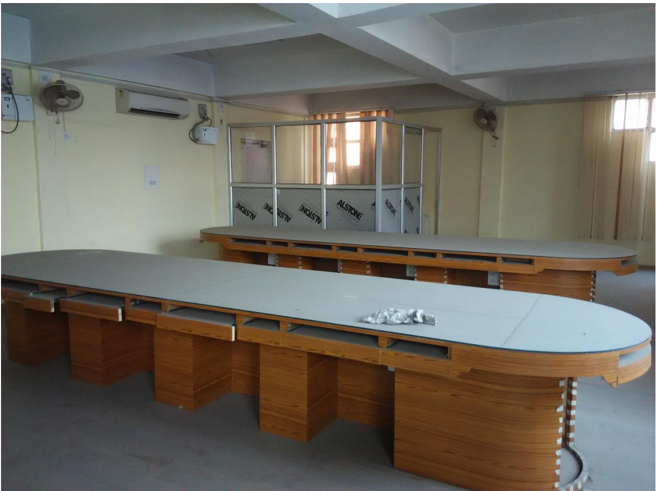
Under construction Computer Lab on the 1 st floor of IMPARD Main Block, Srinagar
